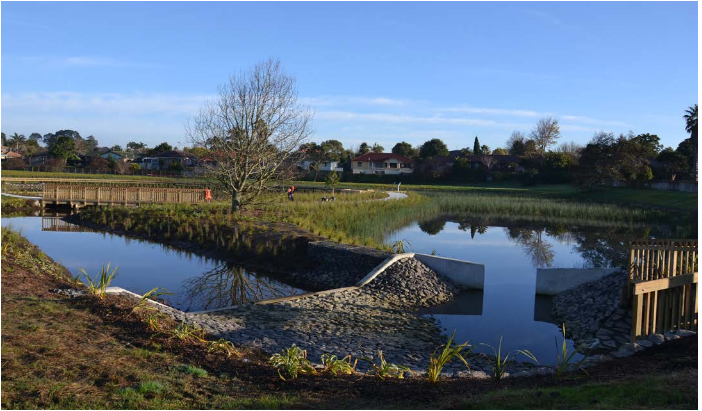
Figure 9: Inlet to constructed wetland showing diversion from online channel to wetland forebay. Brylee Reserve, Auckland.
